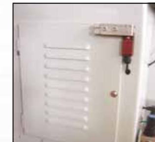
Power off device (door unclose)
